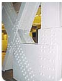
Building truss four-hour rated with AlbiClad TF, at MTA
