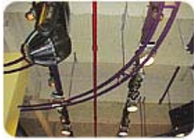
Exposed fireproofing in a retail store. Product by Southwest Vermiculite Type 5.
