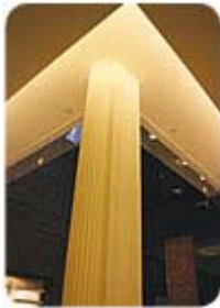
Ornamental steel column with intumescent fireproofing, made by AD Firefilm II, applied at Bloomingdales department store in Soho, New York.
