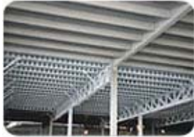
A combination of castelated ("smart beams") and wide flange steel beams with high-density fireproofing Cafco Fendolite M II, from Solatek, at The Grand Avenue Bus Facility, Queens.
