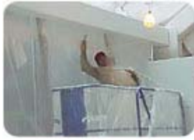
Fireproofing contractor applying intumescent fireproofing at the New York Hilton Health Club. Material supplied by AlbiClad TF.
