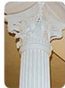
Ornamental column with AD Firefilm II intumescent fireproofing at Bloomingdales.
